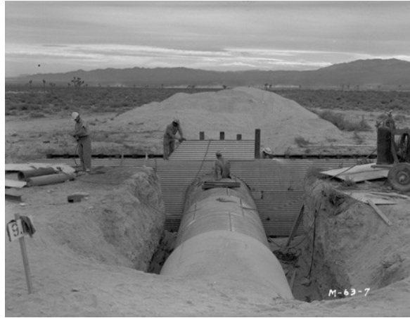
Communal shelter with steel construction, BUSTER {9.1b}
